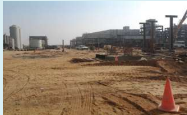
DAHSOUR COMPRESSOR STATION
